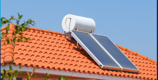
Solar Water Heating
